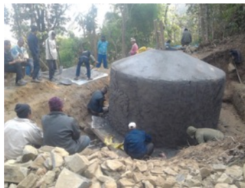
Holding tank for potable water
